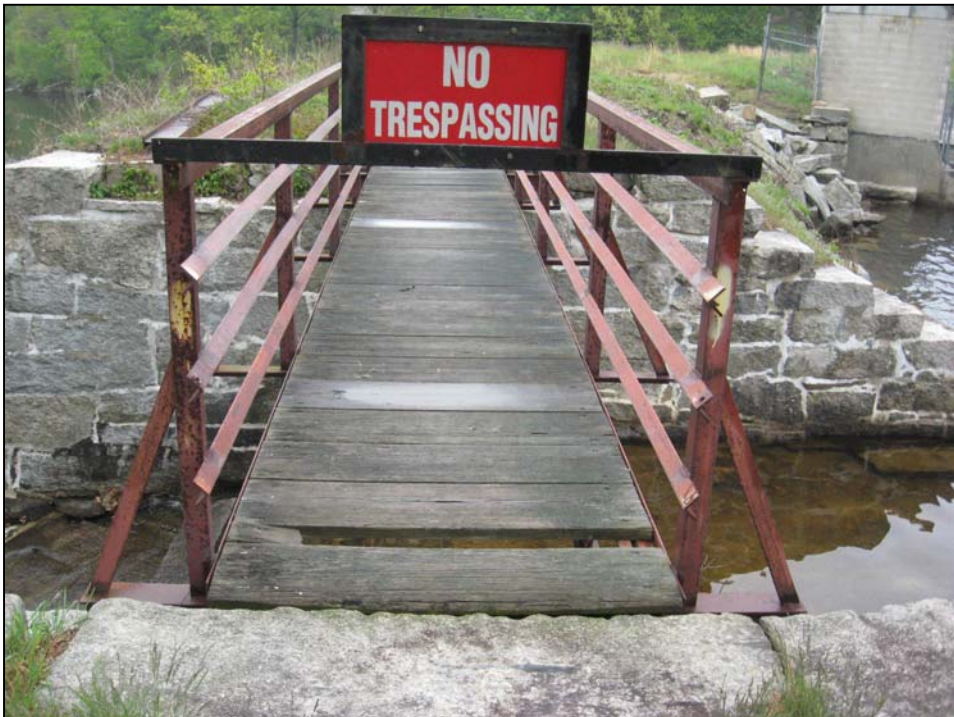
Photo No. 18: Footbridge over the primary spillway looking right. Note broken board.
