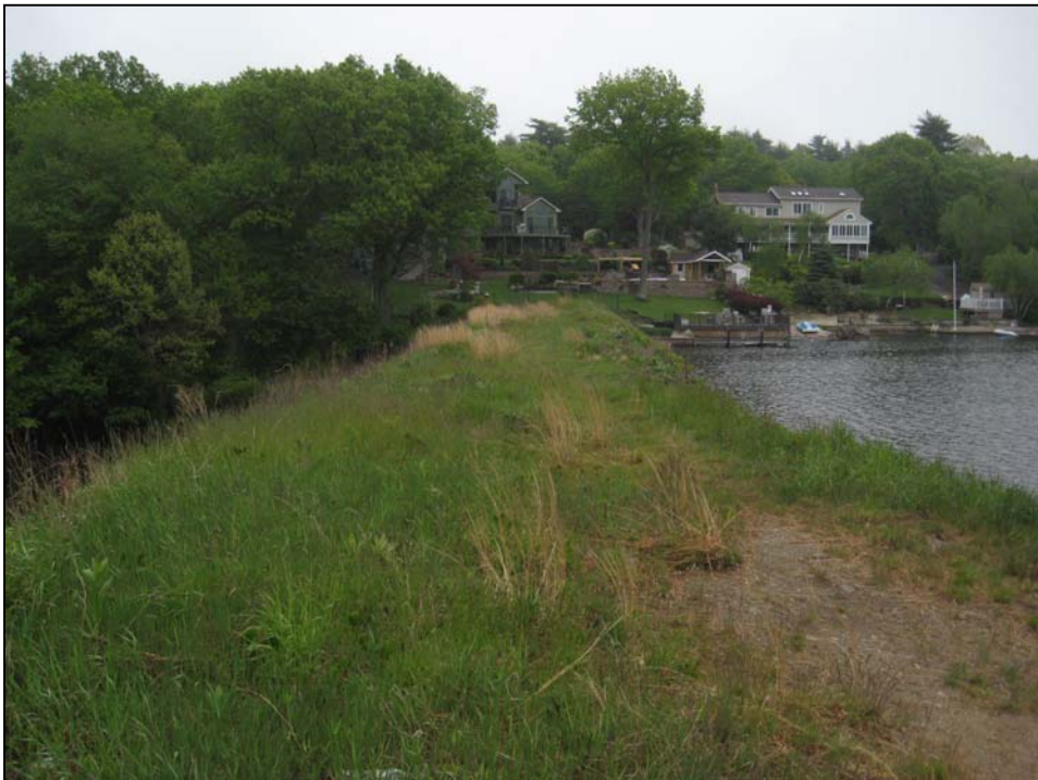
Photo No. 8: Overview of crest from the alignment of the low level outlet looking right.
