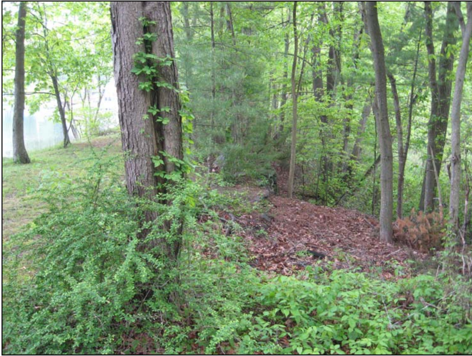
Photo No. 33: Overview of downstream side of the west dike as viewed from the dike's right abutment.
