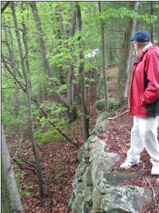
Photo No. 34: Overview of downstream wall of the west dike as viewed from about halfway across the dike looking right.
