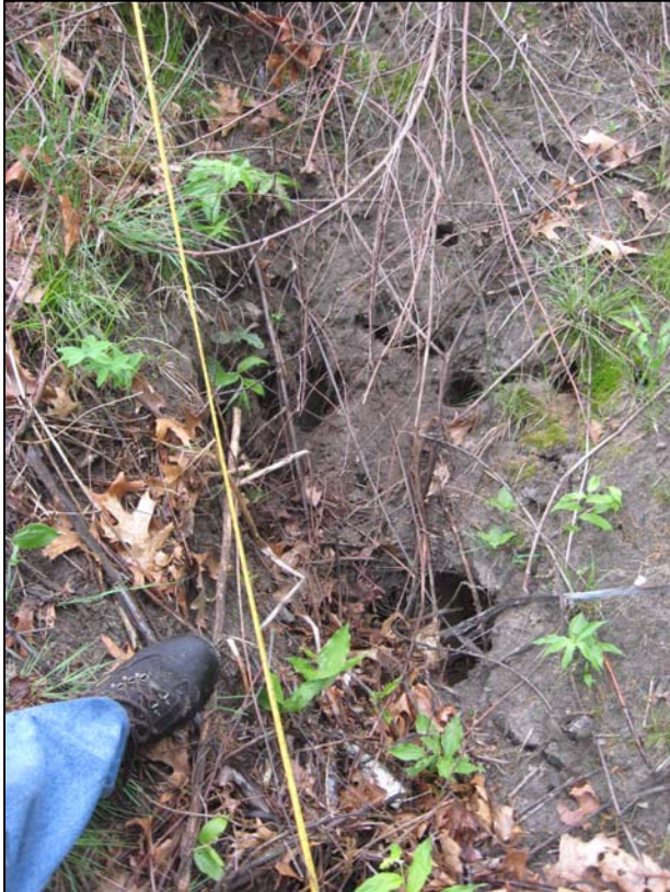
Photo No. 13: Closer view of the large hole observed behind the left downstream training wall to the primary spillway. Note a root mat obstructs the true size of this hole.
