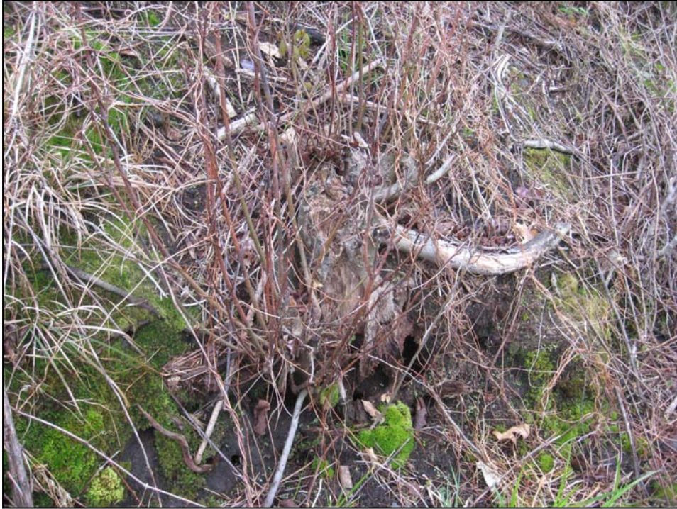
Photo No. 17: Typical rotted stump along based of downstream slope (Photo taken near Station 2+50).
