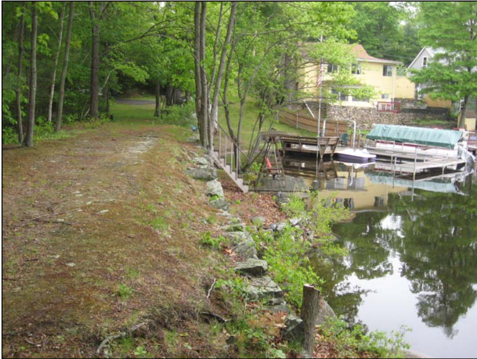
Photo No. 27: Overview of upstream side of the west dike as viewed from Station 0+60 looking right.
