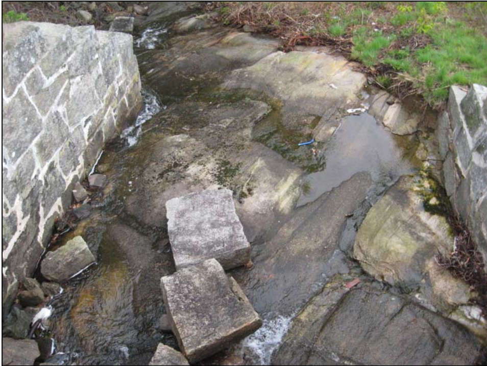
Photo No. 19: Downstream channel to primary spillway. The granite blocks in the channel were removed from the spillway crest as part of previous work.
