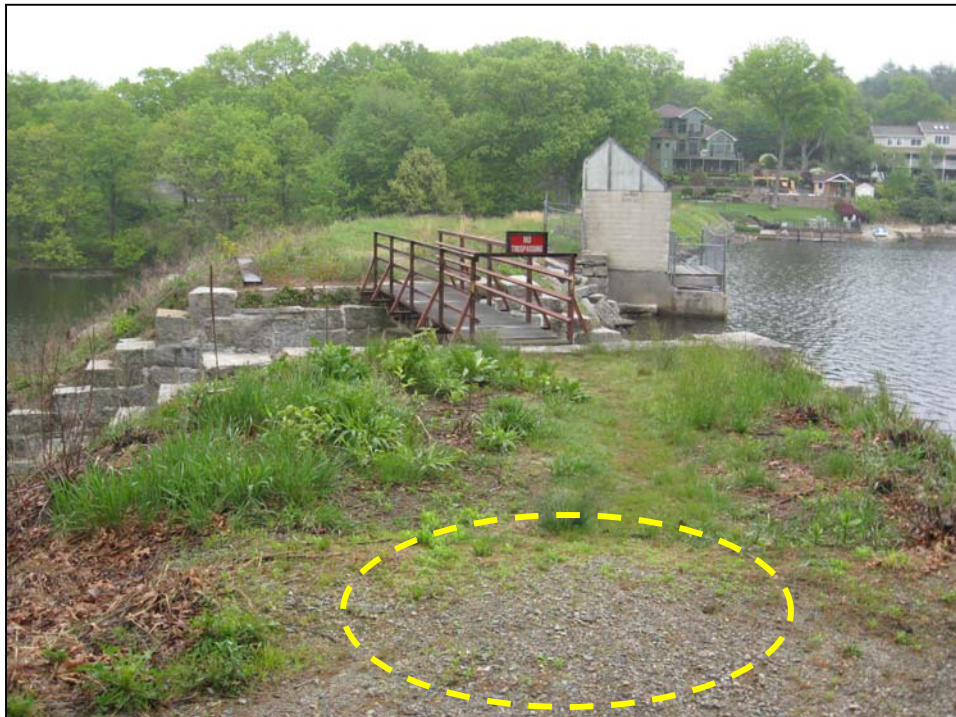
Photo No. 6: Overview of crest in area of the primary spillway looking right. Note eroded area possibly due to foot traffic.
