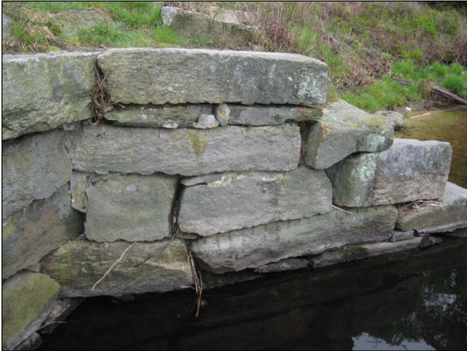
Photo No. 23: Left downstream training wall to low level outlet. Note gaps and movement in wall.
