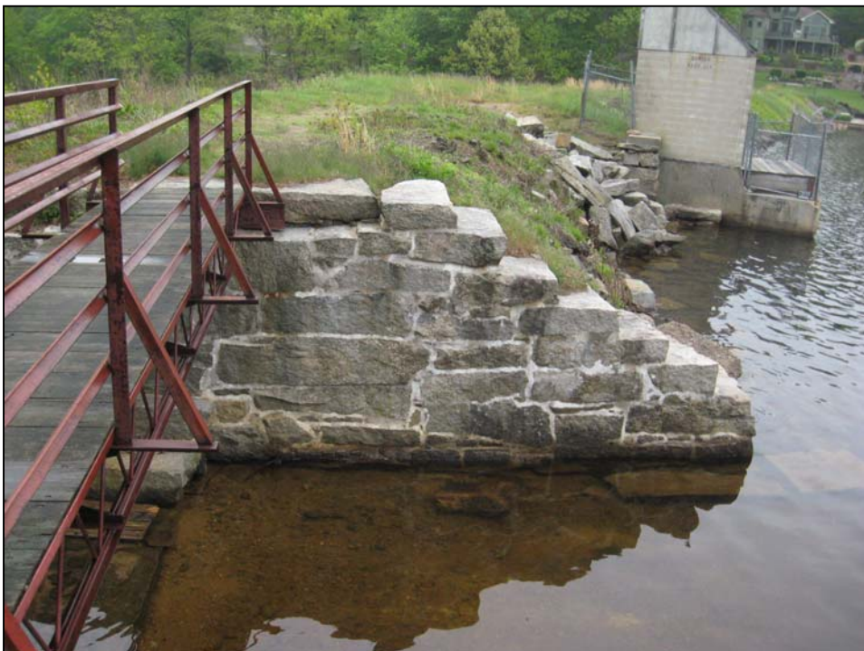
Photo No. 20: Overview of the right upstream training wall to the primary spillway. Note newly mortared joints.
