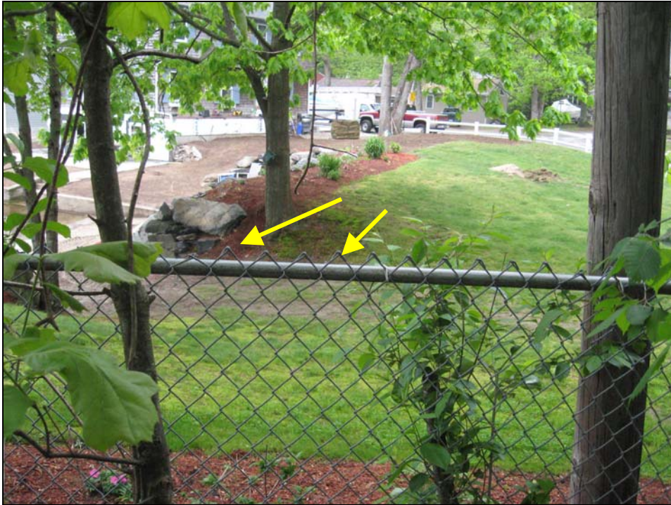
Photo No. 31: Overview of left abutment along the crest of the west dike. Note lower area.
