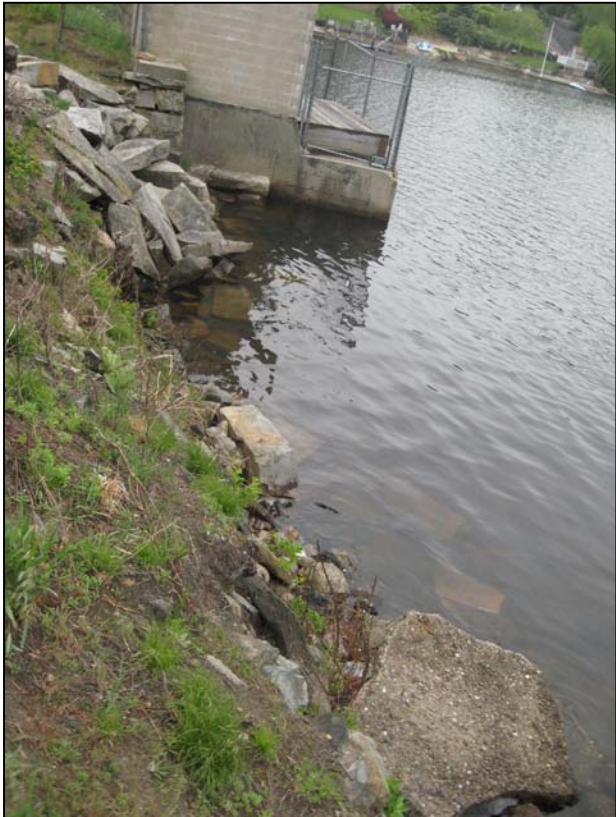
Photo No. 3: Erosion of the upstream slope left of the low level outlet.
