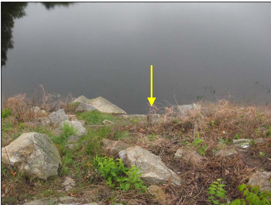
Photo No. 22: The discharge end of the low level outlet as viewed from the crest looking downstream.
