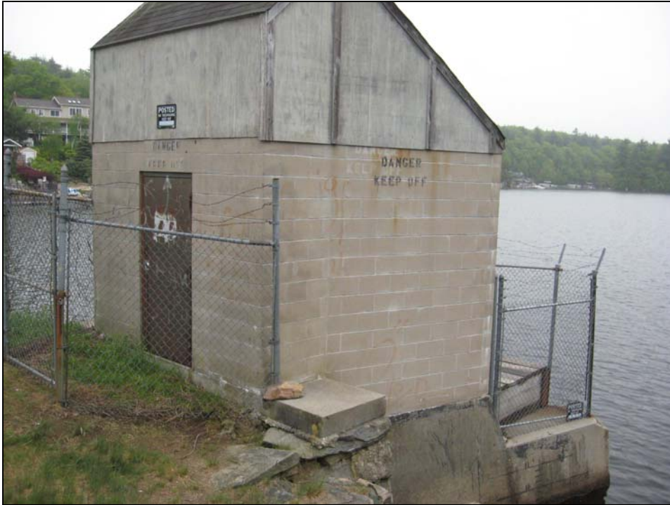
Photo No. 21: The control structure to the low level outlet.
