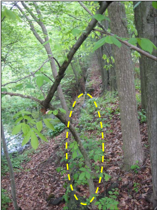
Photo No. 35: Section of failed downstream wall of the west dike as viewed from Station 0+40 looking right.
