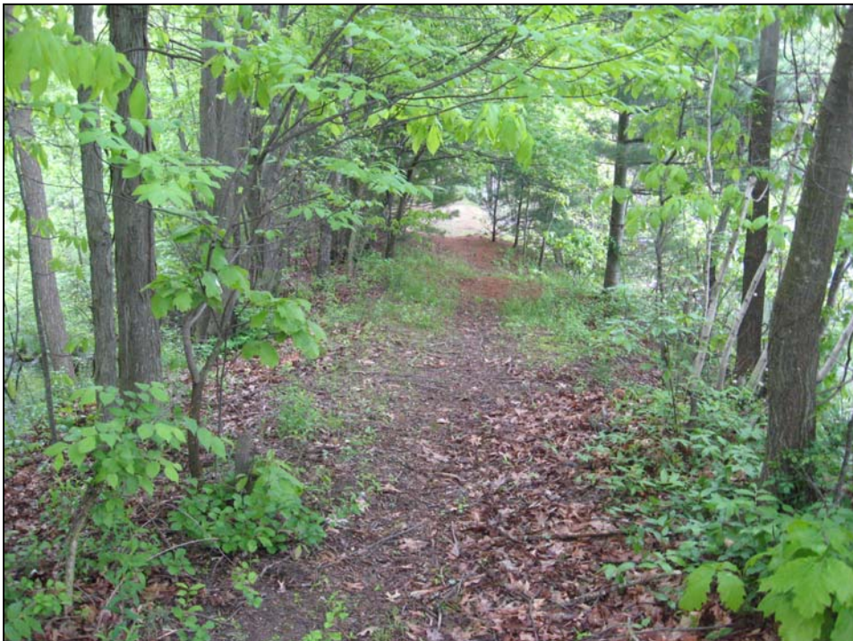
Photo No. 32: Overview of crest of the west dike as viewed from the dike's left abutment.
