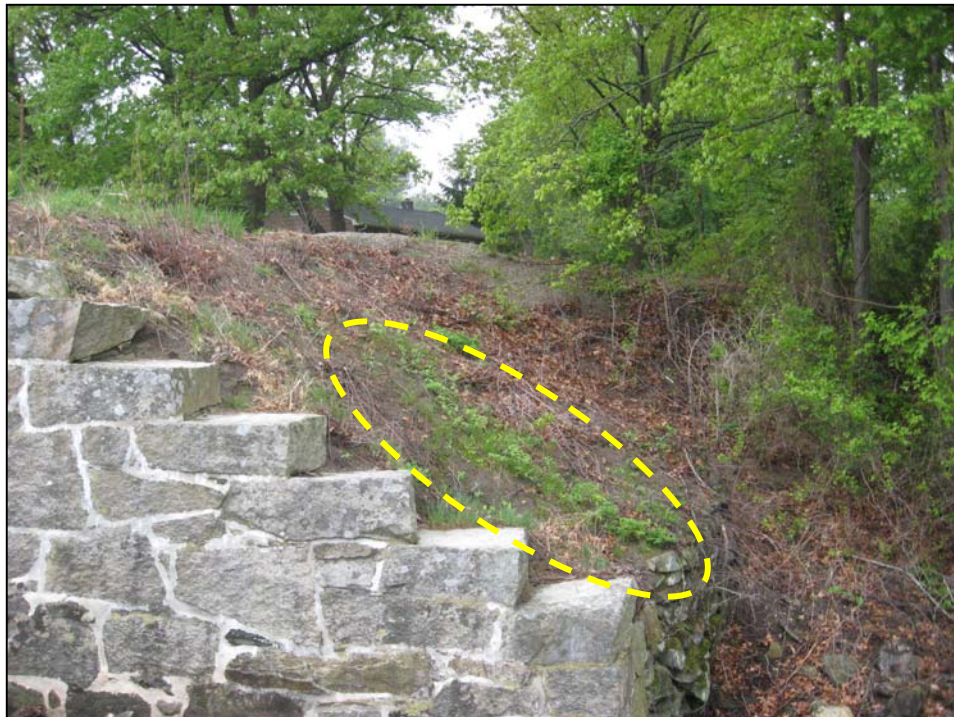
Photo No. 12: Overview of the left downstream training wall to the primary spillway. Note location of large hole (8' L x 3' W x 4' D) observed behind wall.
