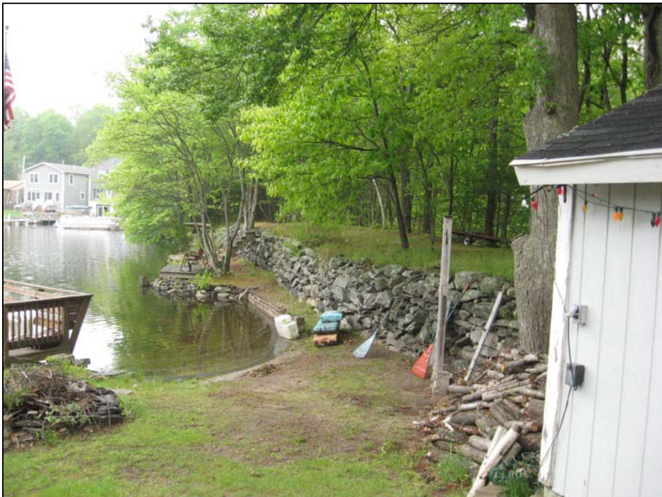
Photo No. 26: Overview of upstream side of the west dike as viewed from the dike's right abutment.
