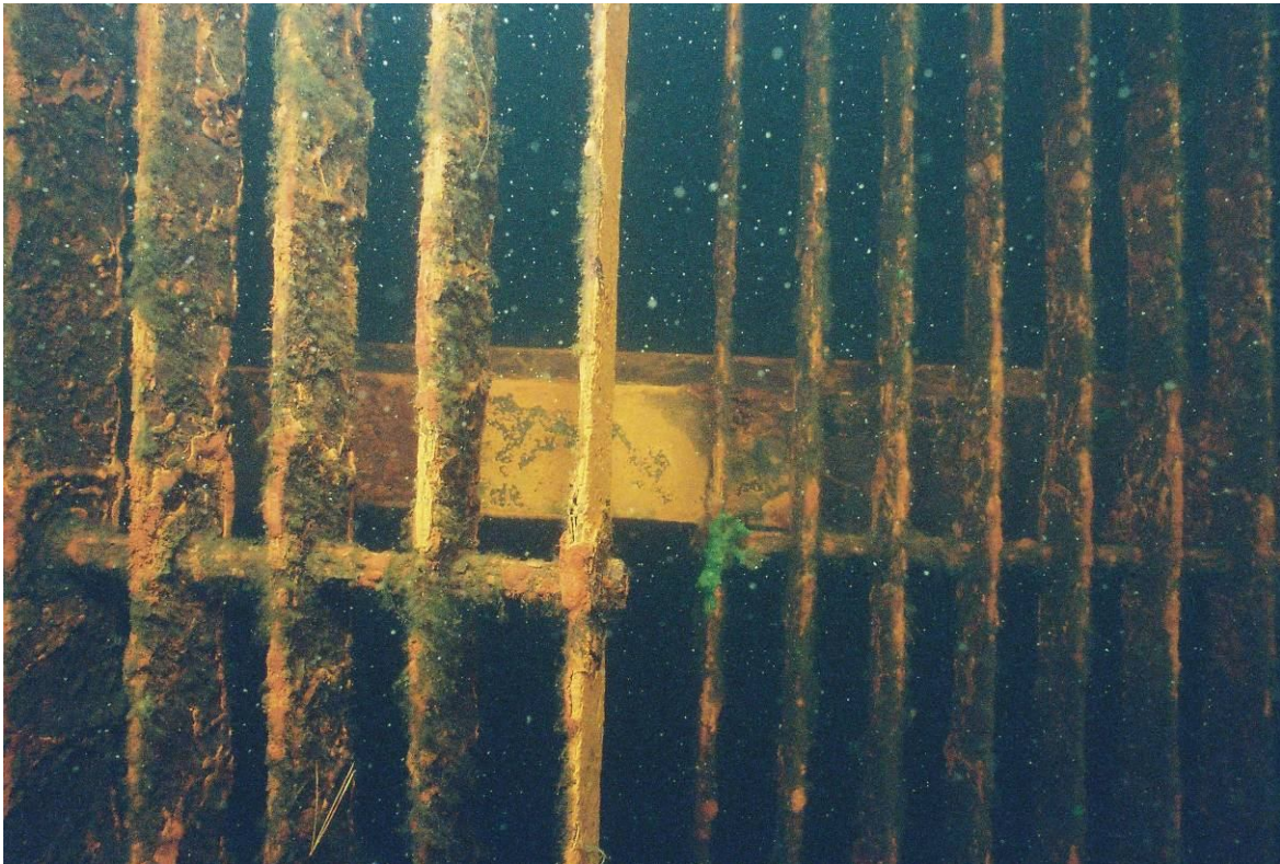
PHOTO #2 SHOWING TRASHRACK DETERIORATION, NOTE HORIZONTAL SUPPORT BEHIND
